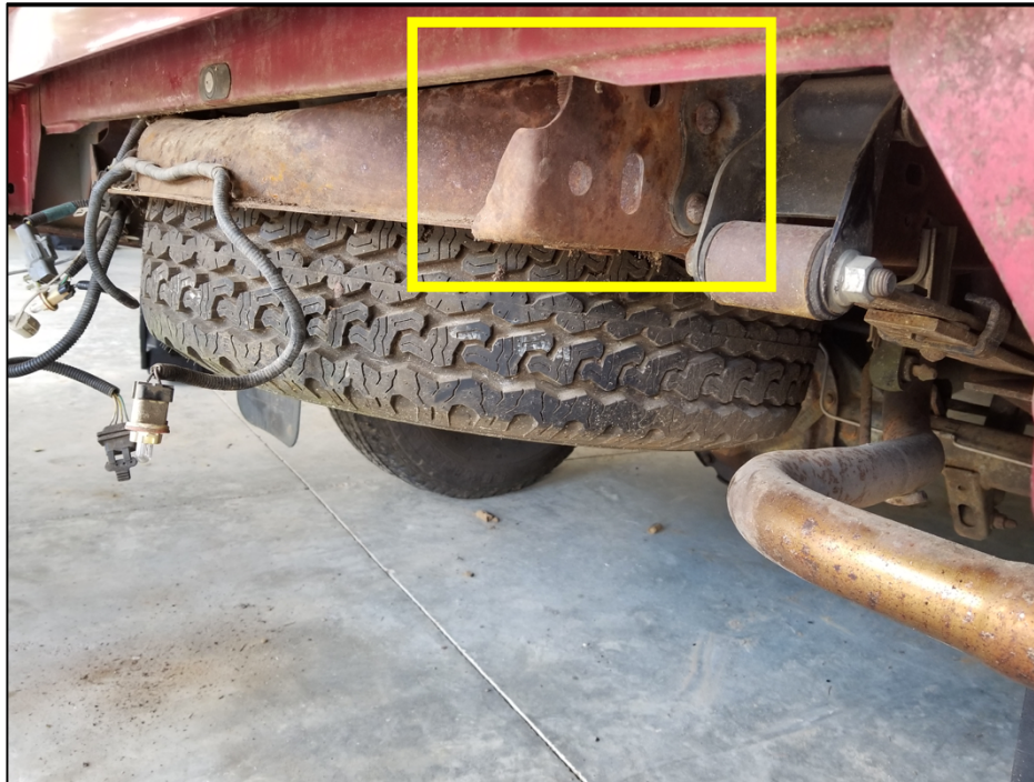
Figure 2. The primary attachment points to the frame are highlighted in this figure. This is an isometric view of the structure shown above.
